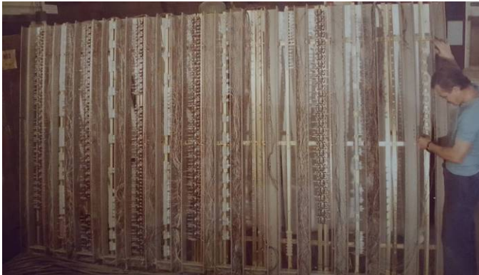
Bornier " raccordement mesures " RAM (partiel)
